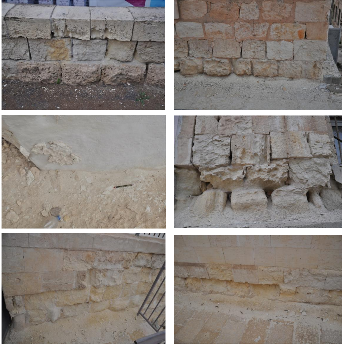
Figure 57: Building stones from the Governor White Unit are sensitive to desert weathering. Rock disintegration causes severe damage to buildings
