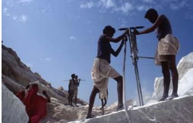
A. Drilling holes with mechanical hammers of ~1 m depth and 20 cm from each other
